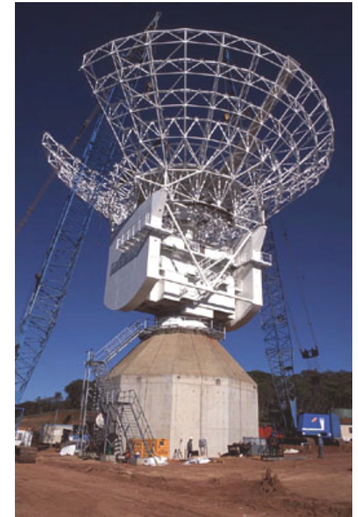
ESA Deep Space Antenna 35m, Ka-band capable
